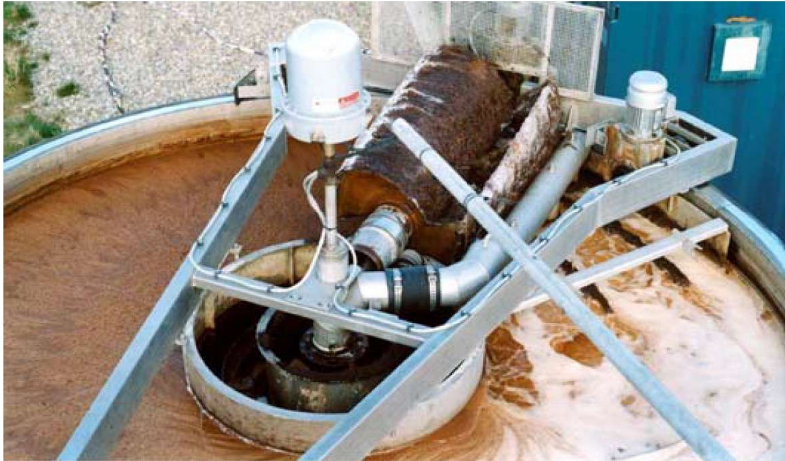
Plate 2.6: The main DAF treatment tank at Arpley Landfill
