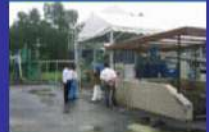
Mechanised Dewatering Unit Completed : 23 Nos
