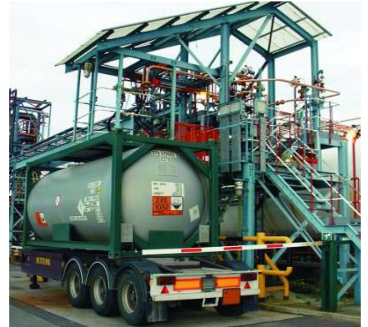
Figure 10 Hydrofluoric acid is a very corrosive liquid. Here it is being loaded automatically into a road tanker.
